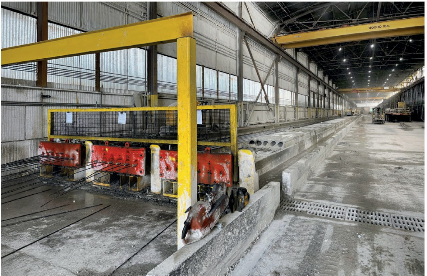
Interior view of the IPS production plant in River Rouge, United States
